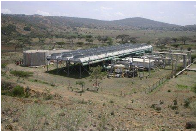
Aluto Langano Power Plant
